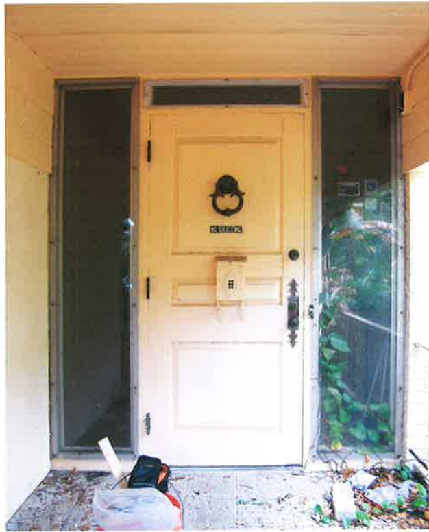
8DB04547: above, altered front porch looking northwest; below, altered entrance looking north.
